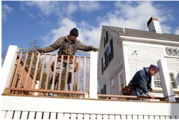
Carpenters Noel Ripley and Dave Thorne build a deck on a home they're renovating in Cohasset, Mass. AF View Enlarged Image
